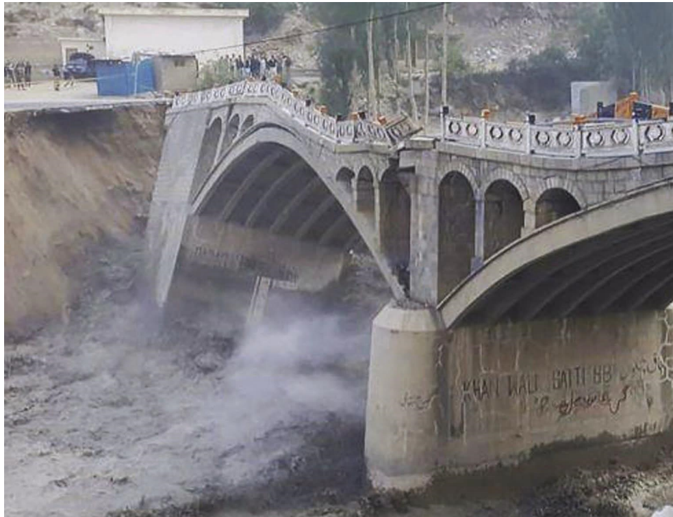
FIGURE 2: Partial collapse of Hassanabad bridge.
